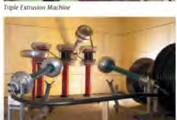
EHV Testing Facility
